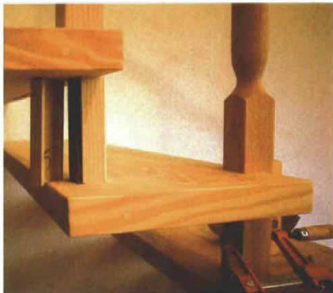
Stealth balusters. Back sections of the balusters are removed, dadoed to conceal the metal bracket and then reattached. Special care was taken to match the cutoff with the correct baluster.
