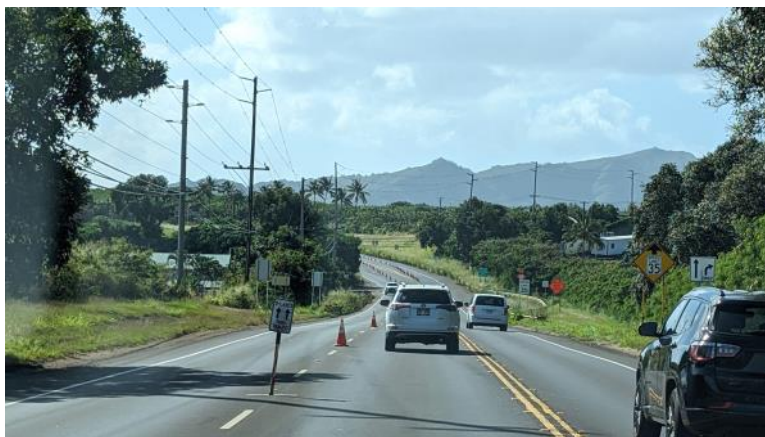
Cones set up to support traffic pattern between Lihue Airport and Kapaa
